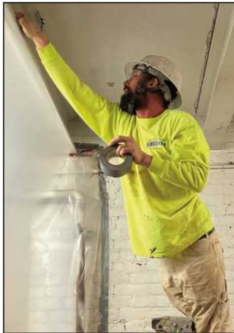
TAPING A PLASTIC BARRIER prior to sandblasting and painting the mechanical room of the Belle Isle Aquarium in Detroit is Casey McLaughlin of Michigan Painters District Council Local 1052. He's employed by Murray Painting.
