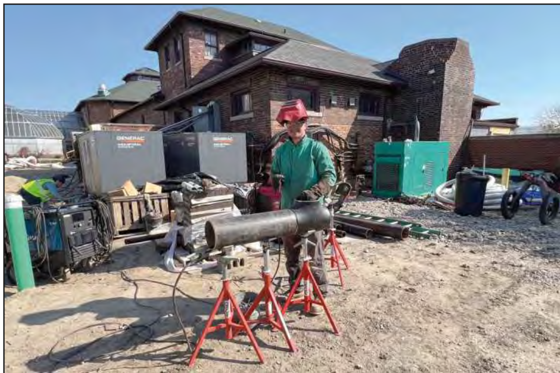
IN THE PROCESS of dismantling and moving an access ramp to the Belle Isle Aquarium in Detroit is Elijah Evans of Laborers Local 1191. He's employed by Christman Constructors.
