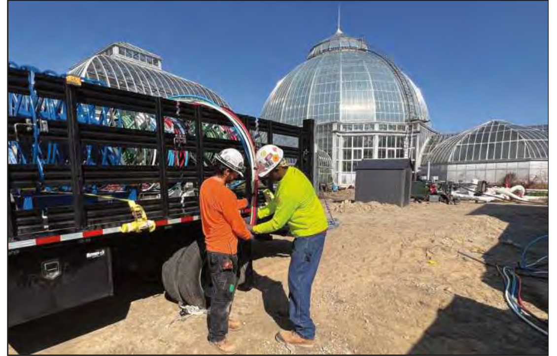
UNCOILING 600 KCMIL GENERATOR wire at the Belle Isle Aquarium project in Detroit are electricians Nick Gross and Leonard Robinson. The IBEW Local 58 members are employed by W.J. O'Neil. Behind them and next door to the aquarium is the magnificently restored Anna Scripps Whitcomb Conservatory, which also opened in 1904.
