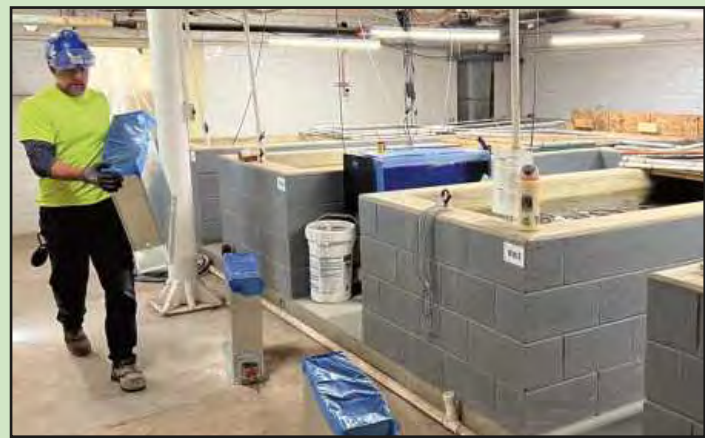
HEFTING DUCT WORK that will feed forced air to the gallery above at the Belle Isle Aquarium is Don Jones of Sheet Metal Workers Local 80. Beside him are fish holding tanks. He's employed by Forced Air Systems, Inc.
