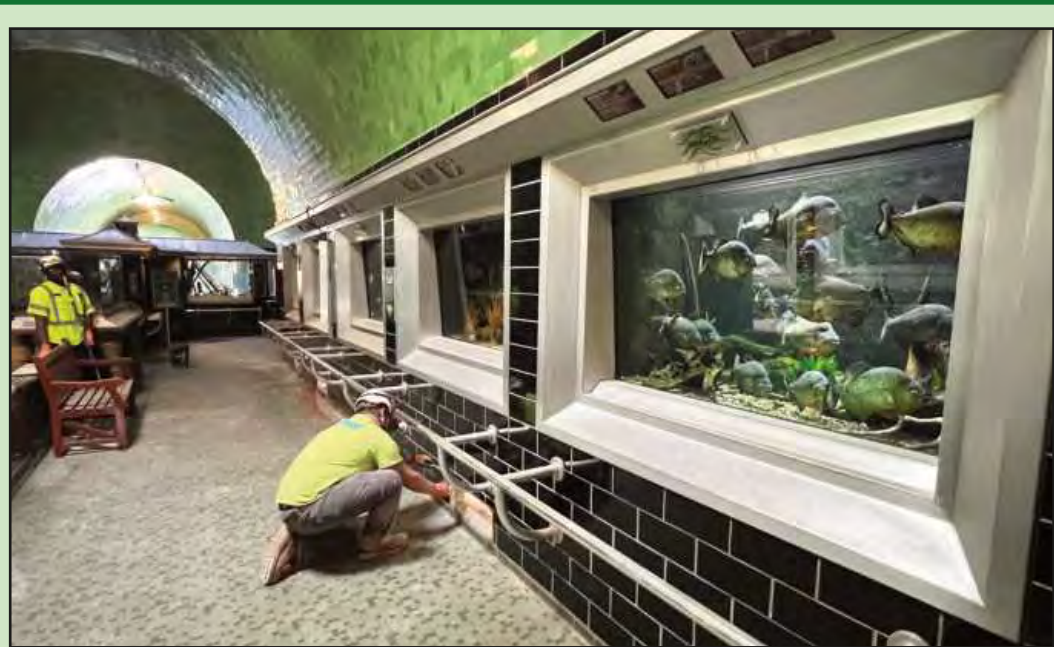
TUCKPOINTING around a new HVAC duct opening in the gallery of the Detroit Aquarium on Belle Isle is Ryan Dahl of Bricklayers and Allied Craftworkers Local 2 He's employed by Ram Construction Services. Taking little notice at right is a tankful of piranhas. According to the Belle Isle Conservancy, architect Albert Kahn intended for the fish tanks to be framed, like art hanging on the wall in a gallery. The aquarium was one of the largest in the world when it opened in 1904. The Christman Co. is managing an extensive renovation of the building, mainly focusing on HVAC work and foundation improvements. More photos – See Page 12.
