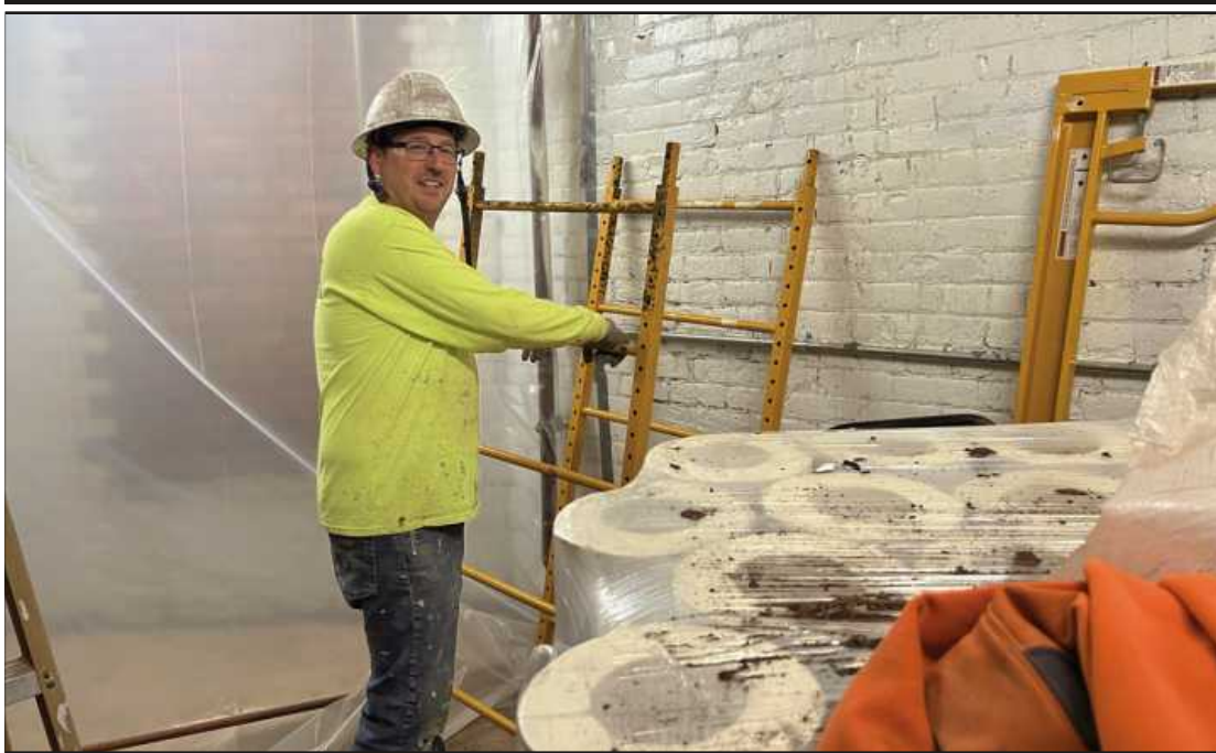
MOVING SCAFFOLDING at the Belle Isle Aquarium project in Detroit is Wayne Marr of Michigan Painters District Council Local 1052. He's employed by Murray Painting.
