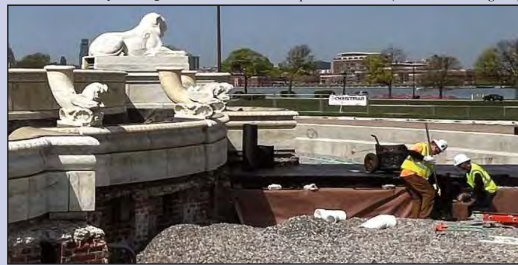
TEMPORARILY ABSENT its main marble basin, the James Scott Memorial Fountain's supporting structure is getting some much-needed improvements during the ongoing renovation project. Here Joe Hubbert and Tommy Burditt apply hot tar to waterproof a portion of the substructure. The Roofers and Waterproofer's Local 149 members are employed by Schreiber Roofing.
