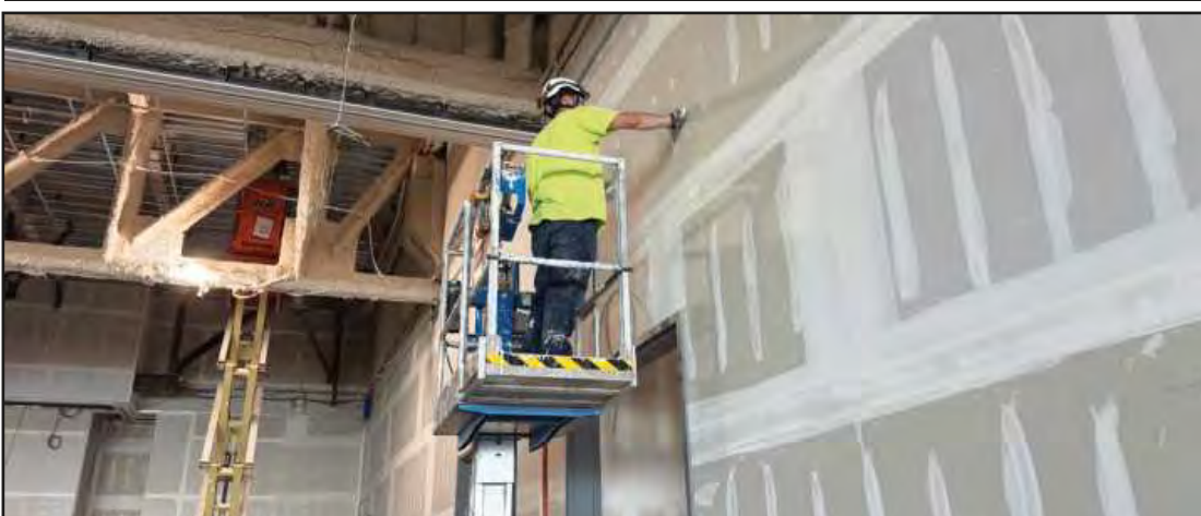
SANDING DRYWALL seams in the junior ballroom at the JW Marriott Detroit Water Square hotel project is Francisco Martinez of Michigan Painters District Council 1-M. He's employed by Brinker.
