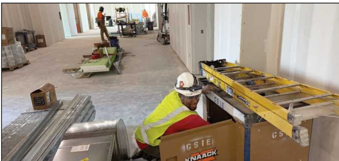
IT'S IN HERE SOMEWHERE: Electrician Eshon Flowers of IBEW Local 58 grabs a tool out of a cart while working at the JW Marriott Detroit Water Square hotel project. He's employed by GSIE.
