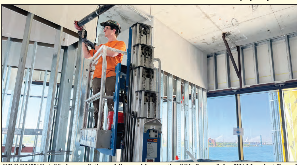
GROOVING A 90-degree fitting while working on the fifth floor of the JW Marriott Detroit Water Square hotel is Nate Weaver of Sprinkler Fitters Local 704. He's employed by Johnson Controls.
