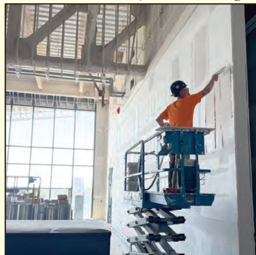
MUDDING DRYWALL seams in the "Junior Ballroom" at the JW Marriott hotel in Detroit is William Minoek of Michigan Painters District Council Local 2352. He's employed by Brinker.
