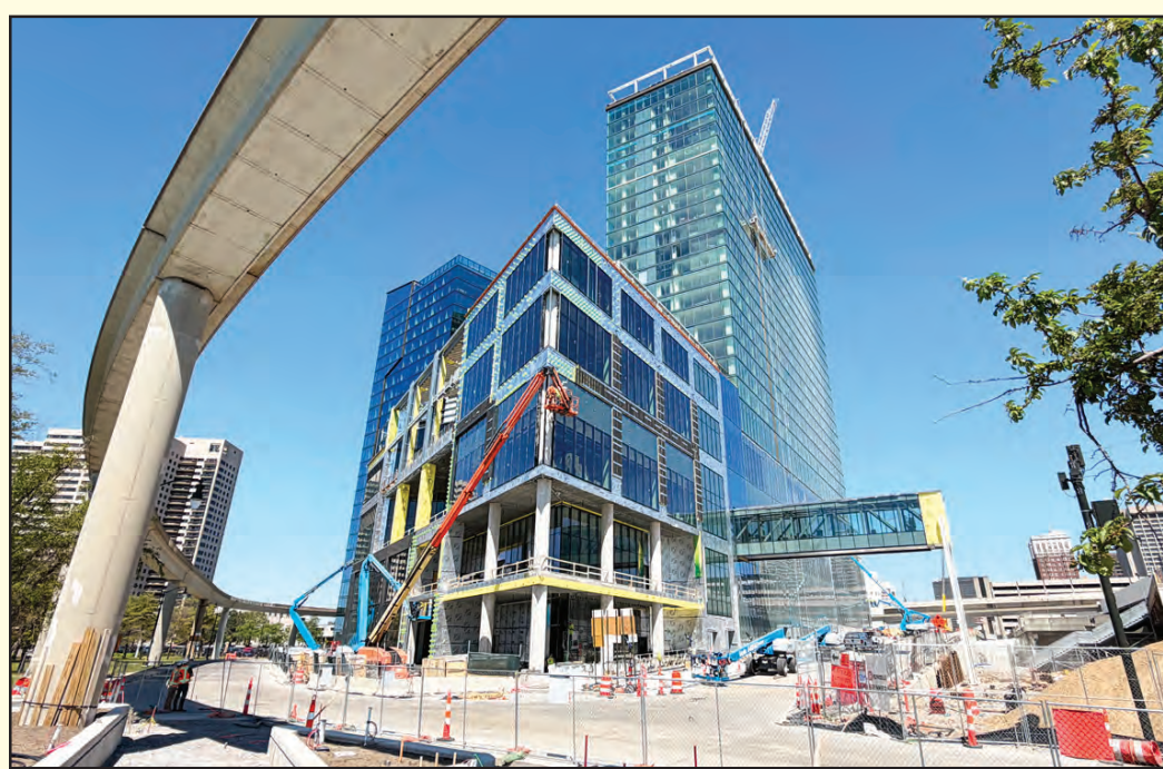
THE 25-STORY JW Marriott Detroit Water Square hotel is being erected on the Detroit riverfront on the former site of Joe Louis Arena. The facility will bring 601 rooms to the city's downtown, and importantly, will provide the first link to the Huntington Place convention center via a skybridge, whose stub is visible at right. Another feature of the project: the skybridge will span a newly extended Second Avenue, which will allow through-traffic from Steve Yzerman Drive on the riverfront to Fort Street.
