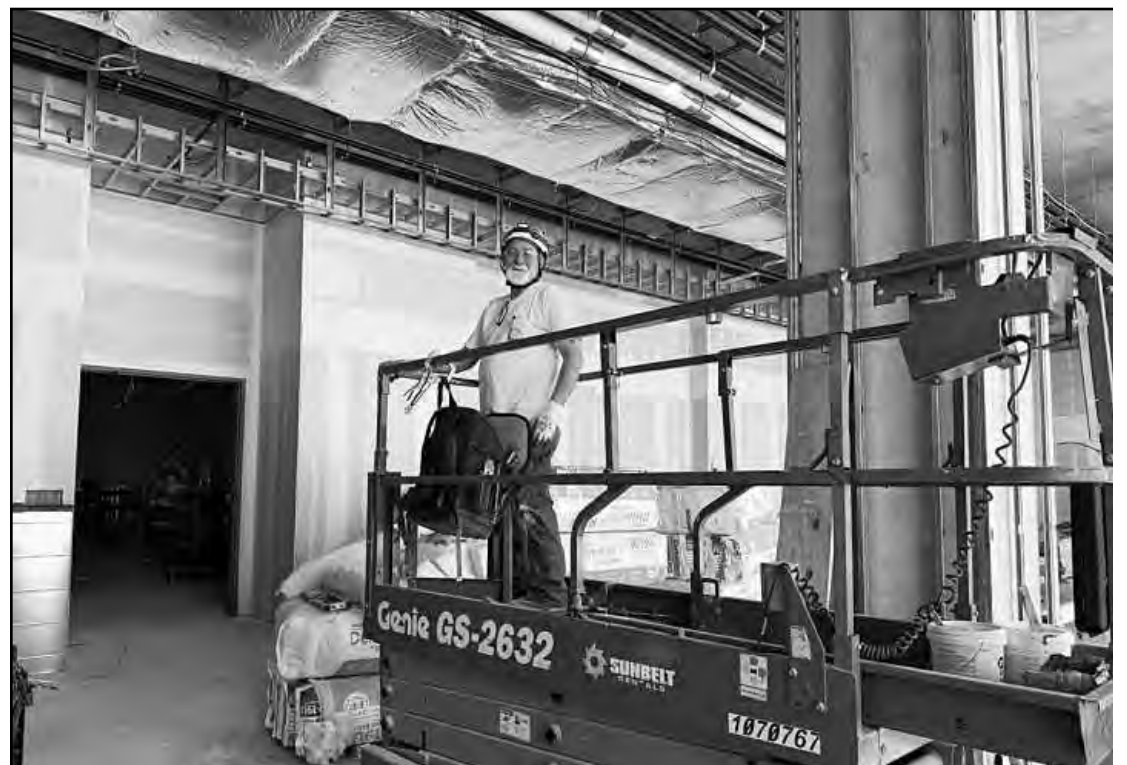
HEADED UP TO WORK on a ceiling duct at the JW Marriott Detroit Water Square hotel project is Jim Roberts of Sheet Metal Workers Local 80. He's employed by Sylvan, Inc.
