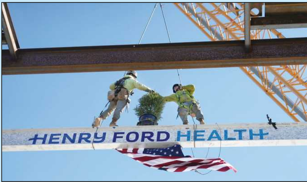
IRON WORKERS Local 25 members set the final 32-foot steel section that will be part of the new patient tower at Henry Ford Health's Destination Grand project.
