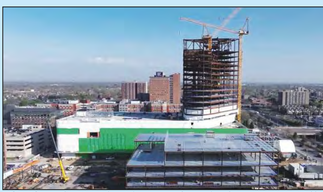
IRON WORKERS and operating engineers set the final section of structural steel on the 20th story of the tower structure at Henry Ford Health's $2.2 billion "Destination Grand" project. Work is proceeding under a joint venture created by Barton Malow, Turner Construction and Dixon Construction. Photo credits: Henry Ford Health
